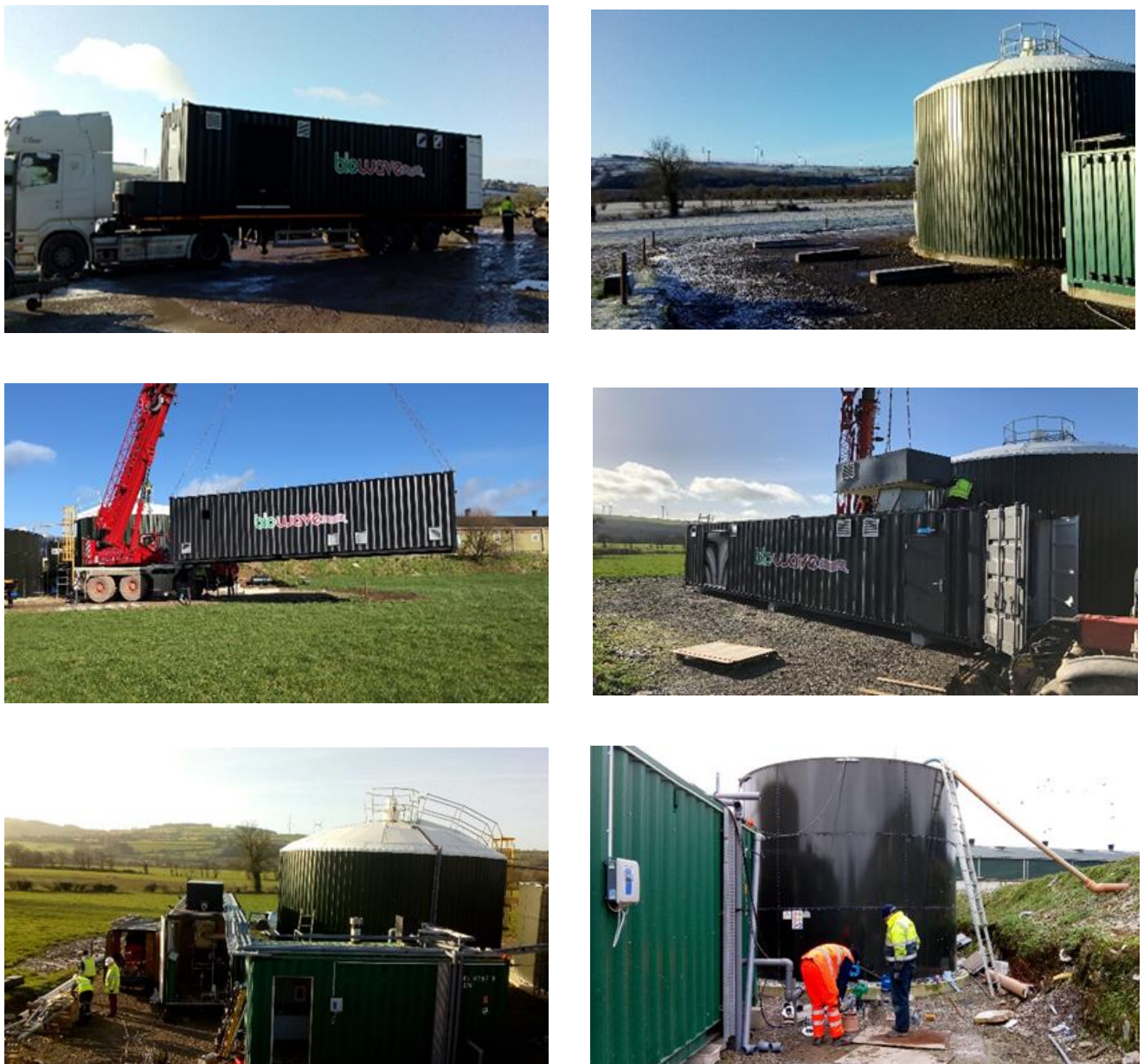
Figure6. Delivery and integration of the Biowave system on Ashleigh Farms
