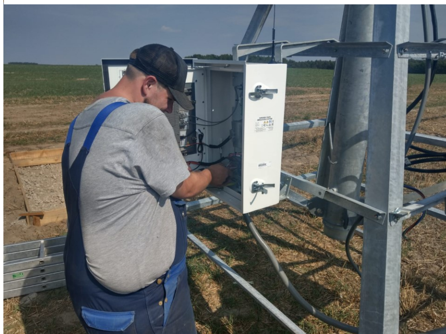
Figure 26 connecting the sub-area controller
