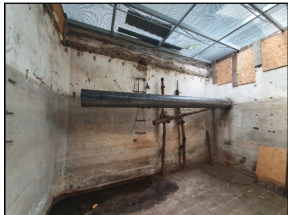
Figure 6 – current pumping station with PVC-Pipe for connection and space for the pumps
