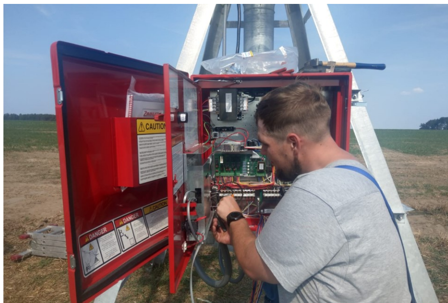
Figure 25 wiring of the main control system
