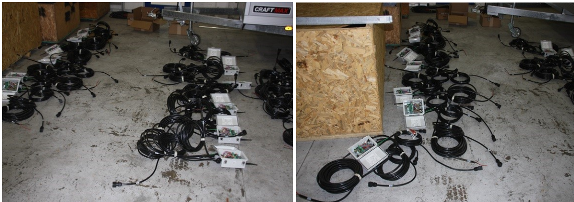
Figure 21 Pre-wiring of the signal nodes
