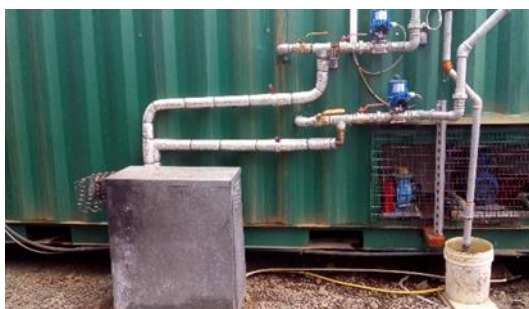
Figure 4. 25 kW oil boiler to augment the thermal energy requirement during commissioning stages.
