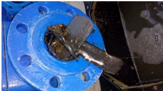
Figure 1. 3- initial blockages in pipework from buffer tank
